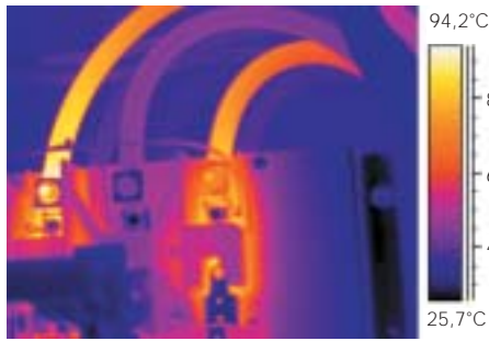
See loose connections
