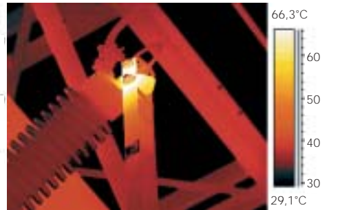
Find incorrectly secured connections
